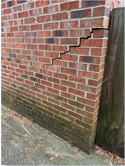
Cracked Corner on Original Wall
